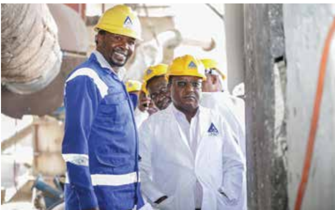
Head of Plant Operations Eng. Stanley Irungu shows Board Chairman Mr. Edwin Kinyua, EBS, the ongoing works inside the Kiln.
