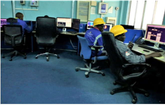
Kiln operators in a busy Central Control Room soon after the recommissioning of the kiln.
