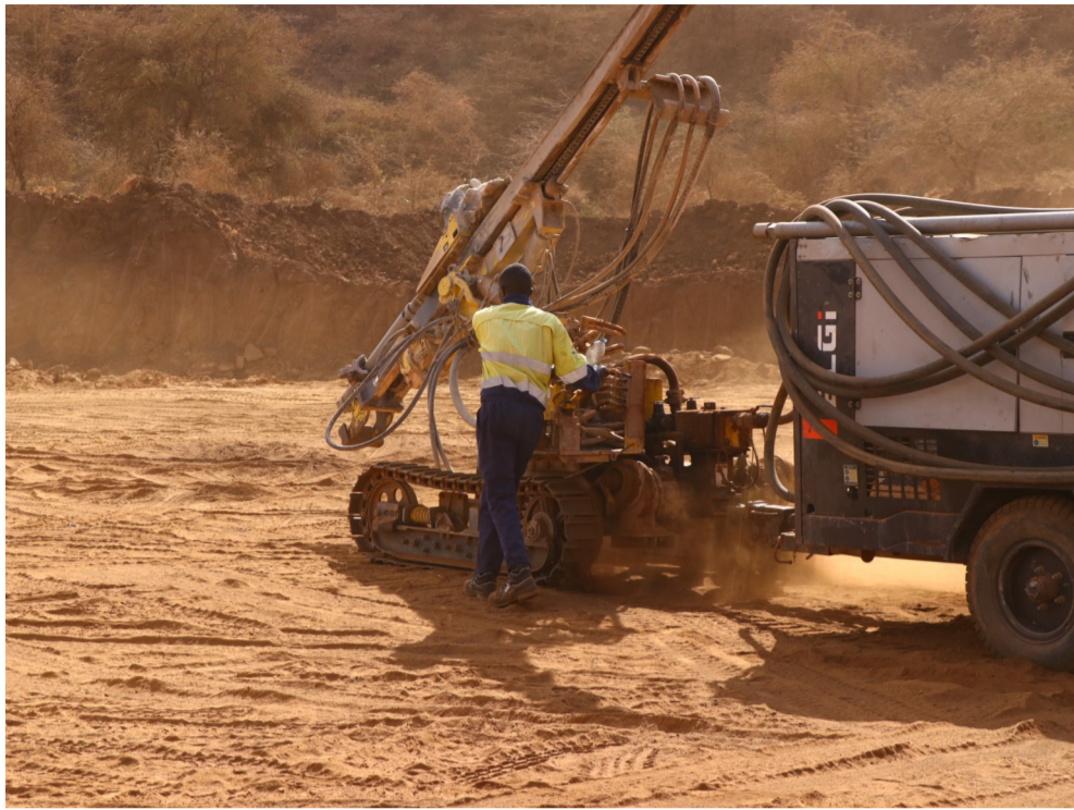
An Operator drills the holes in which explosives are put for blasting
