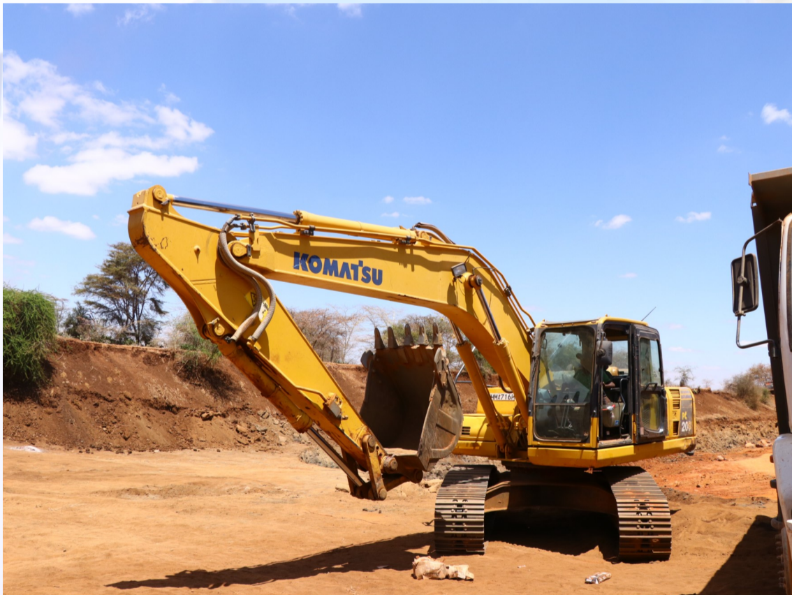
Above: Some of the equipment in use inside the newly commissioned Pit
